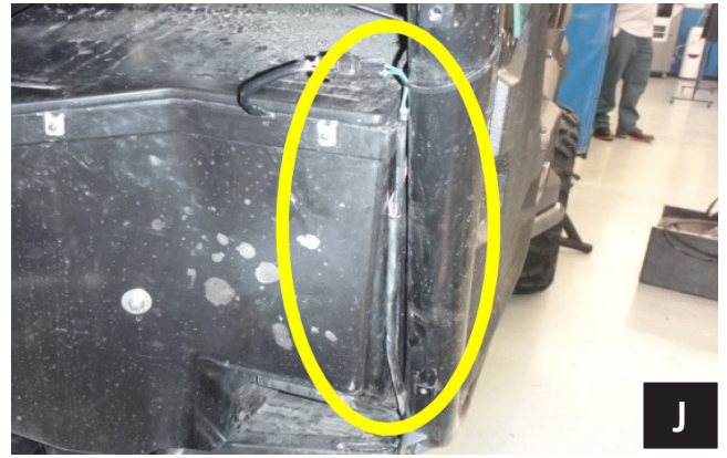
J. Routing the cable down this bar, then under the floor (step K)
